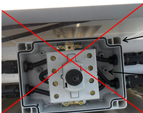
Example of how not to install an isolator.
